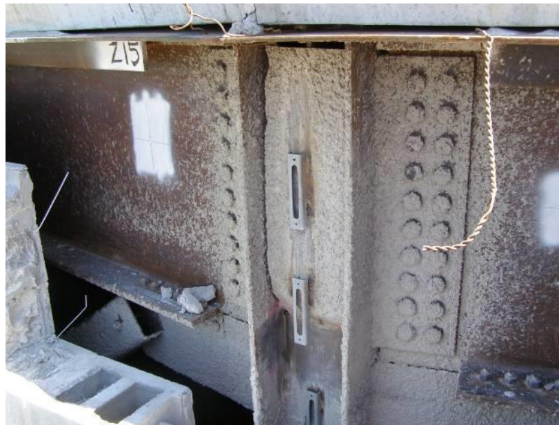
Photo 2: Ruptured Column Web at Dome Tension Ring Connection
